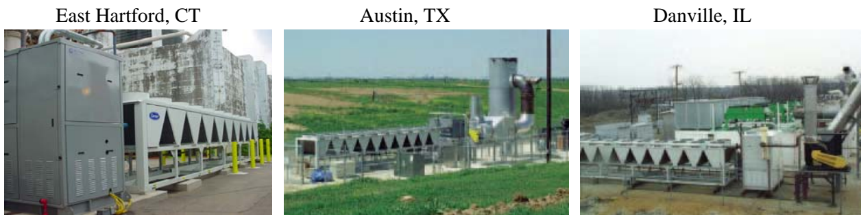
Figure 5. Existing HVAC-derived ORC installation
